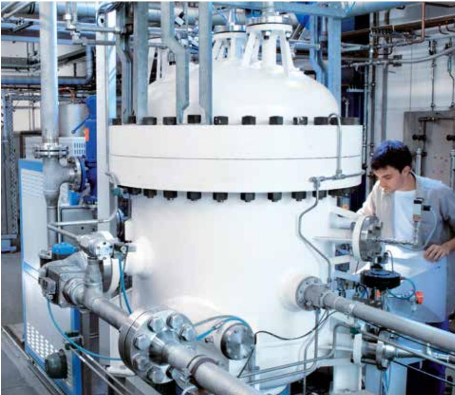
Example of a Carboflex installed heat treatment furnace
