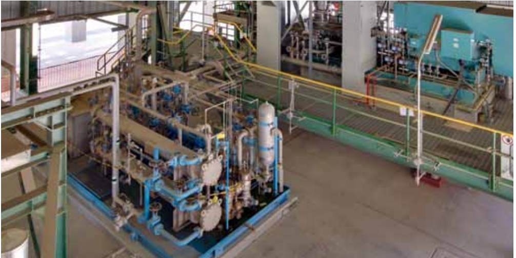
Figure 6: Small membrane separation plant
