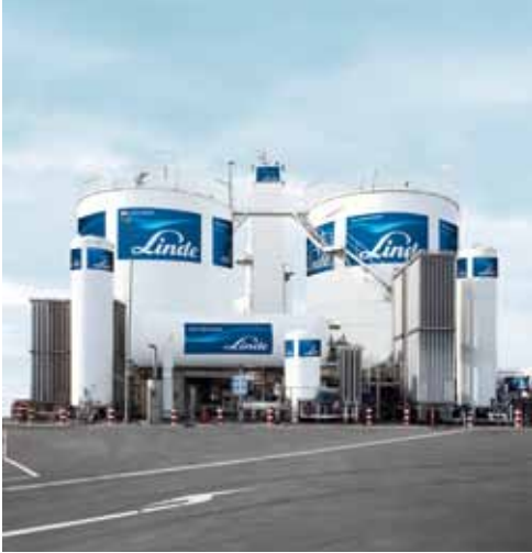
Figure 4: Cryogenic air separation plant
