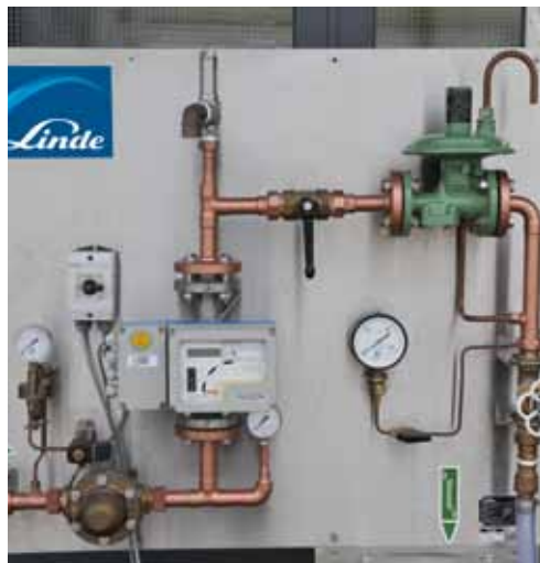
Figure 15: Simple measuring and metering station for the inerting of silos
