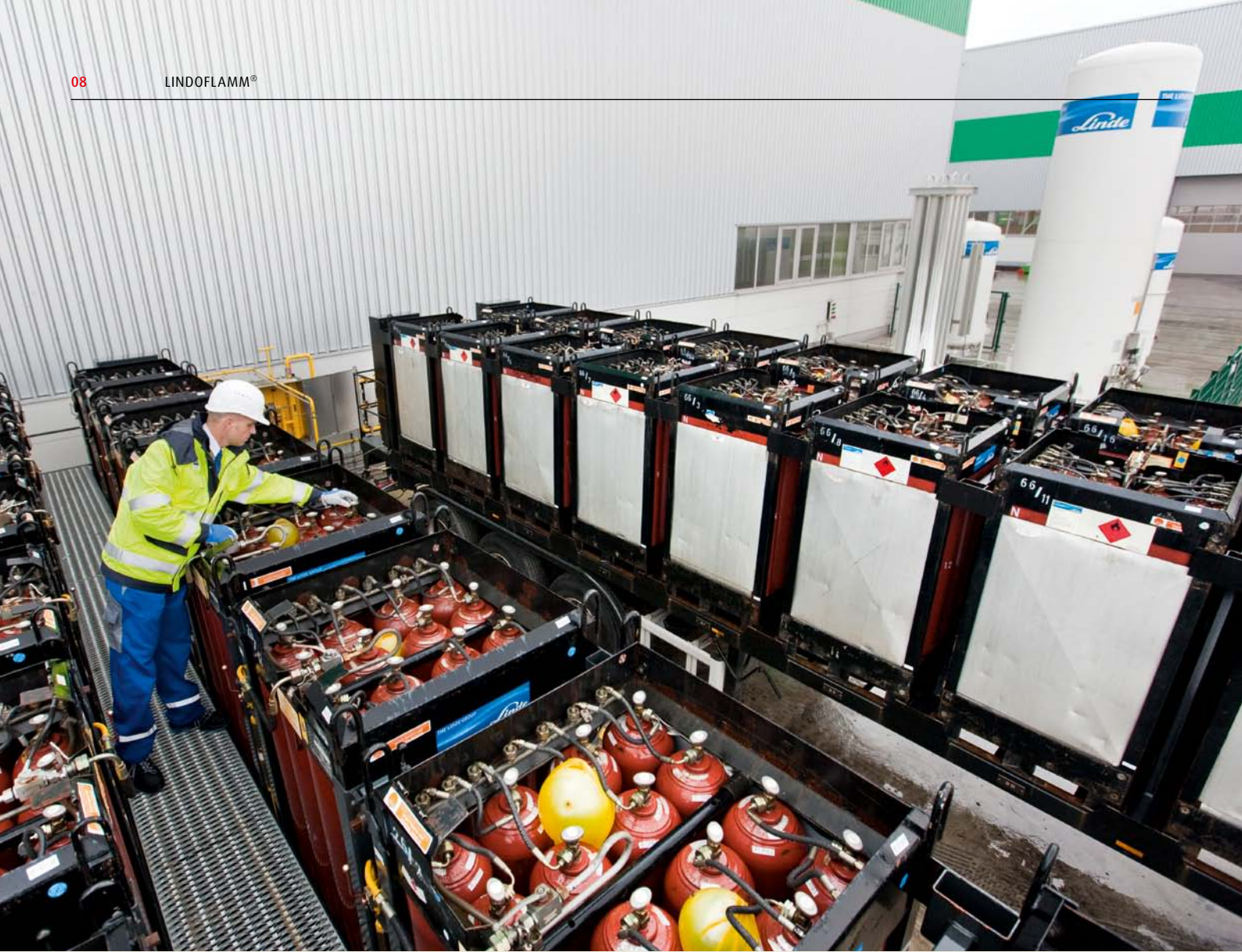
Acetylene trailer packs at a customer in Germany
