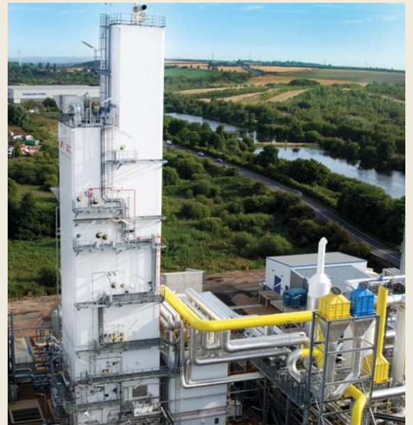
The new Air Separation Unit at Scunthorpe has been built with energy efficiency in mind
