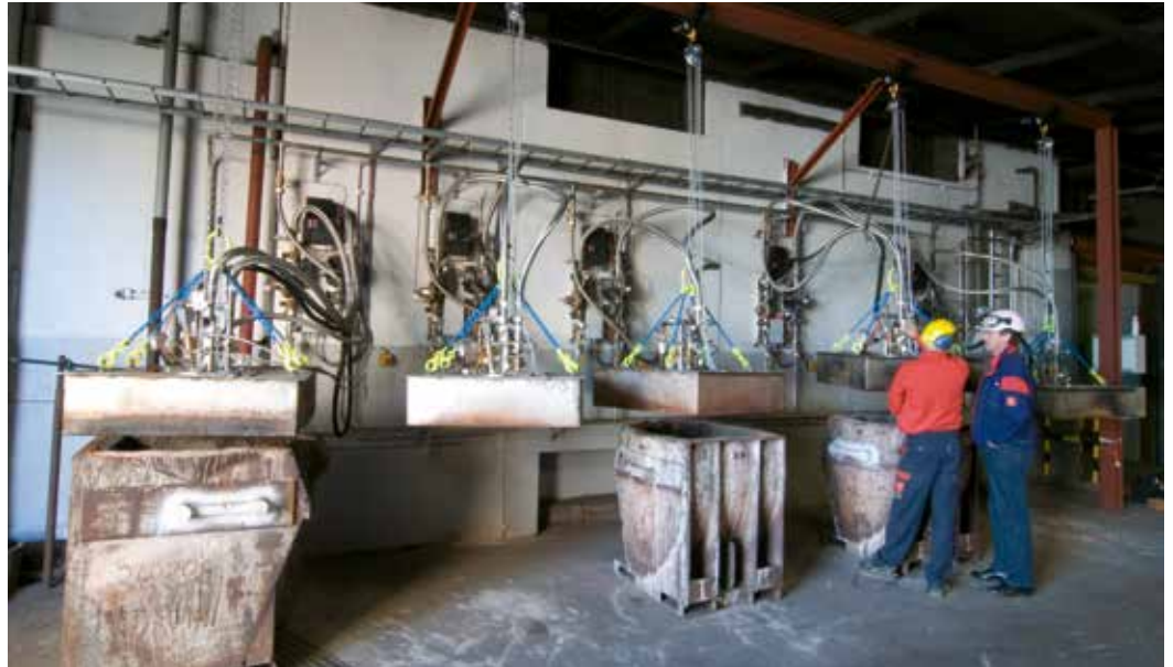
OXYGON® 400 preheating systems installed at SKF in Katrineholm, Sweden; 1 ton ladles are heated in 6 stations.
